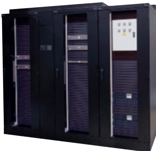
Micro data center solution
